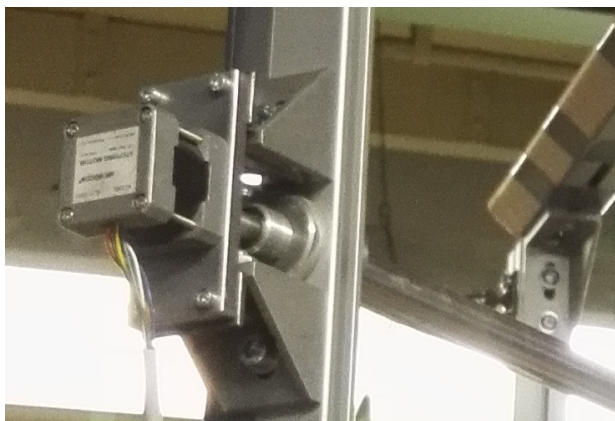
Figure 6: Connection of stepping motor Microcon SL17 - 0301 to axle of rotation at the frame
