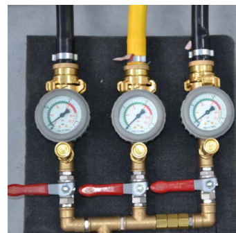
Fig. 12- Valves with pressure gauges
