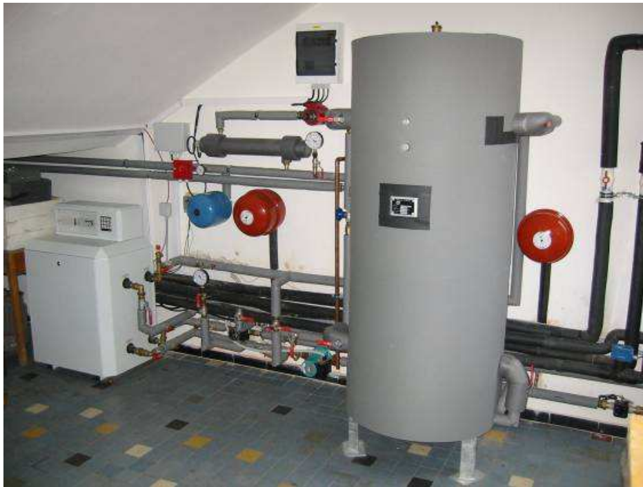
Fig.4: Ground source heat pump system on CTU in Prague, Faculty of Mechanical Engineering
